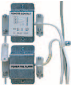
Remote temperature and power failure alarm
